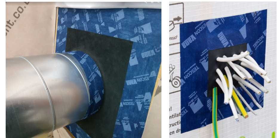
Services entries present a risk to airtightness, however proprietary grommets are available to ensure airtightness can be achieved. The image on the left is of a ventilation duct as a reminder that airtight buildings must have a robust ventilation strategy.
